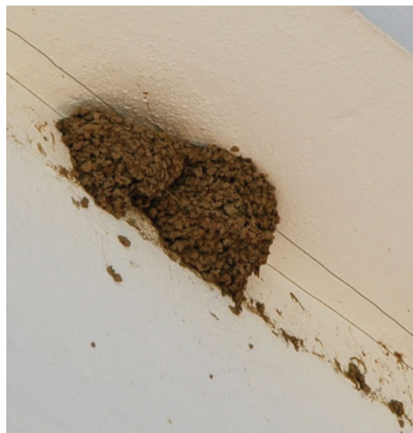
Figure 2. House martin's nest installed on the wires
